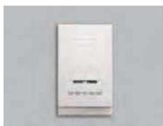
Low Voltage Boxes
