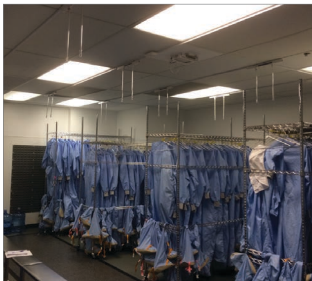
Ceiling Emitters in Gowning Room
